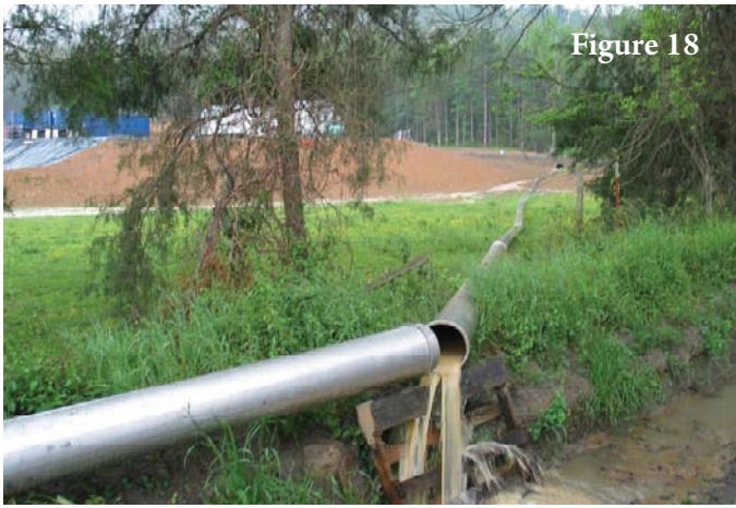
An open pipe leading from a drilling pad discharges into a ditch. The contents of drilling waste is not disclosed to the public.
