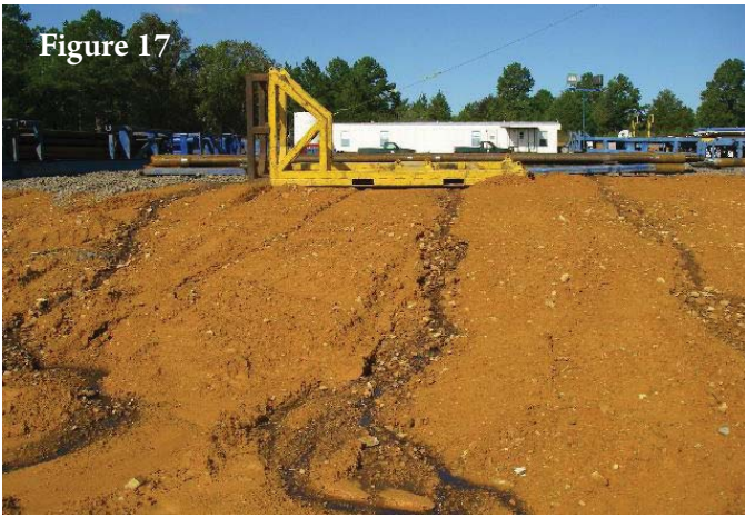
Drilling fluids leaking and running off of a well pad will end up in a nearby lake or stream.
