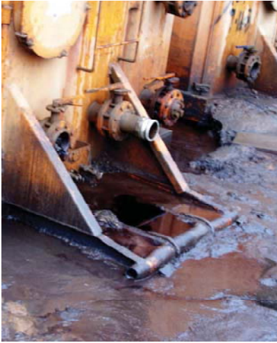
Drilling mud leaking from tanks at a land farm that has since been shut down.
