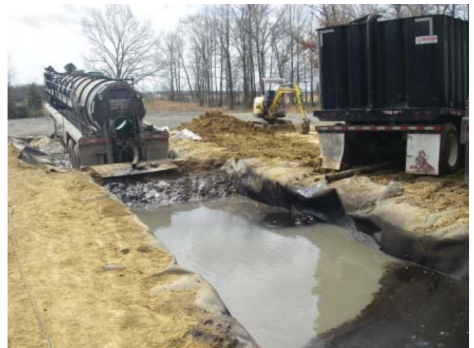
Unpermitted tank and pit storage system.
