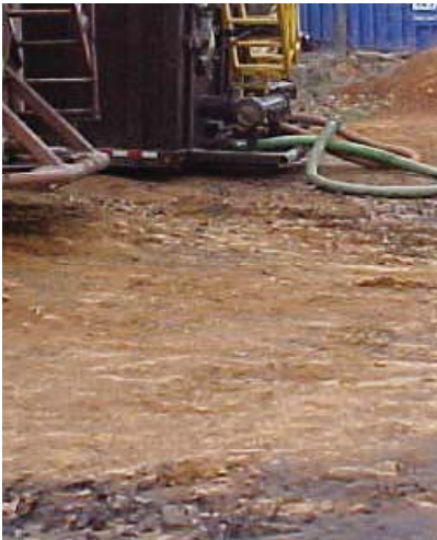
1.11.07 Drilling fluids leaked or spilled on the ground.
