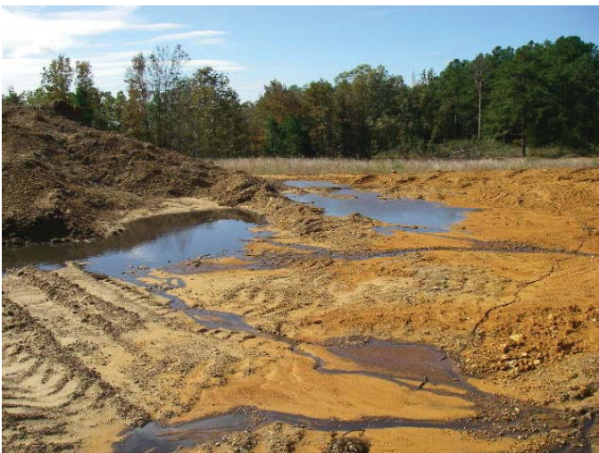
Drilling fluids running off of a well pad. 10.24.07
