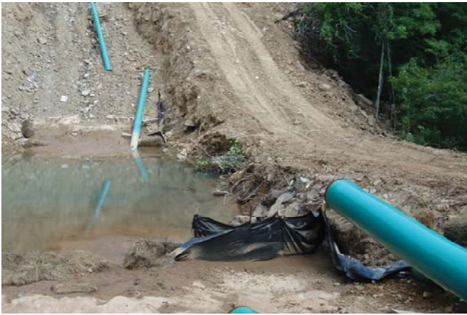
This stream crossing, with downed silt fences and broken pipeline, is contaminated with sediment from previous washouts and has a new road damming the creek with no protection from washing out again.
