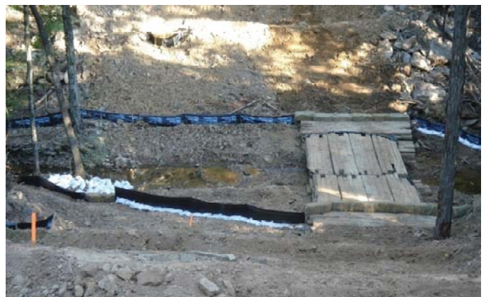
This stream crossing follows Best Management Practices, with silt fences placed parallel to the creek, a bridge that allows water flow and water bars on the slope.
